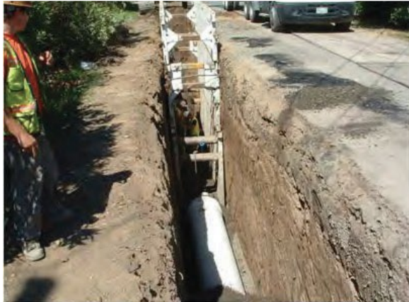
Image of sewer line replacement. Image source: Sonoma Water Capital Improvement Plan 2019-2024
