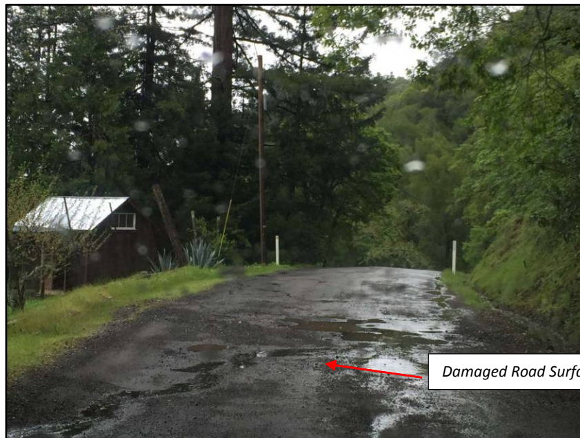
Photo 4 – Damaged Road Surface Condition
