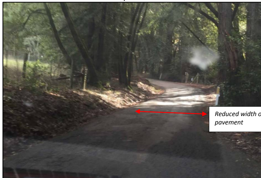
Photo 2 – Narrow Pavement Width
