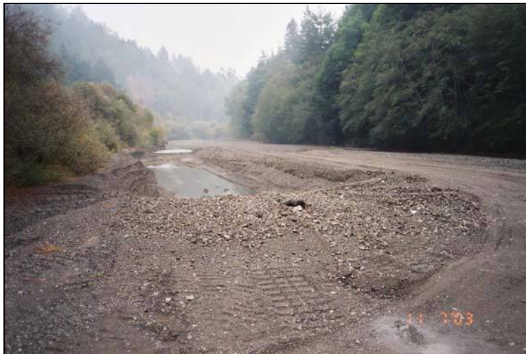
Figure 13. View looking downstream at Bar #2 showing excavated trench in highest part of bar, well away from the low flow channel on the right. November 2003.
