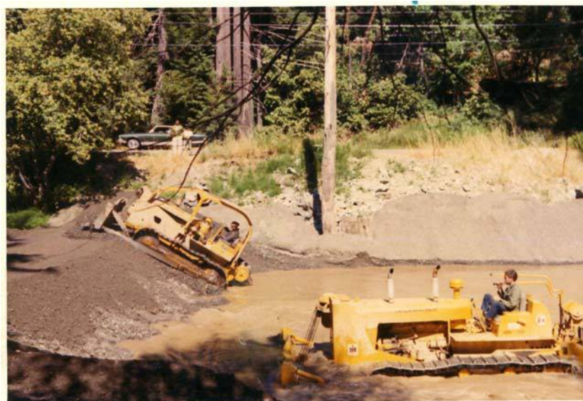
Figure 4. Dozers building a summer dam on Austin Creek, ca. 1970. Source: Homer Canelis.
