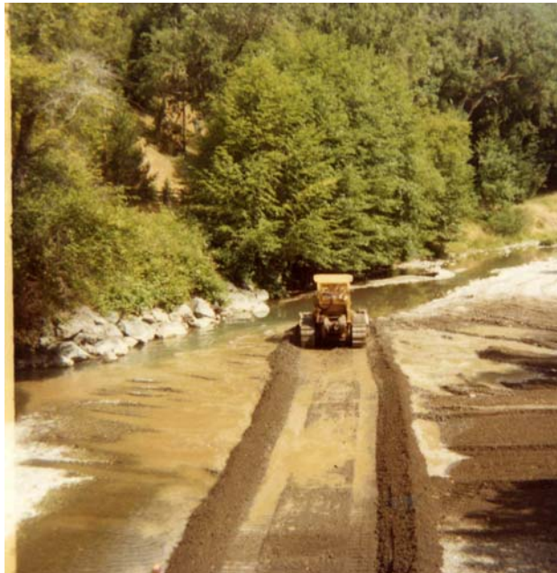
Figure 3. Dozer building a summer dam in Austin Creek, ca. 1970. Source: Homer Canelis.
