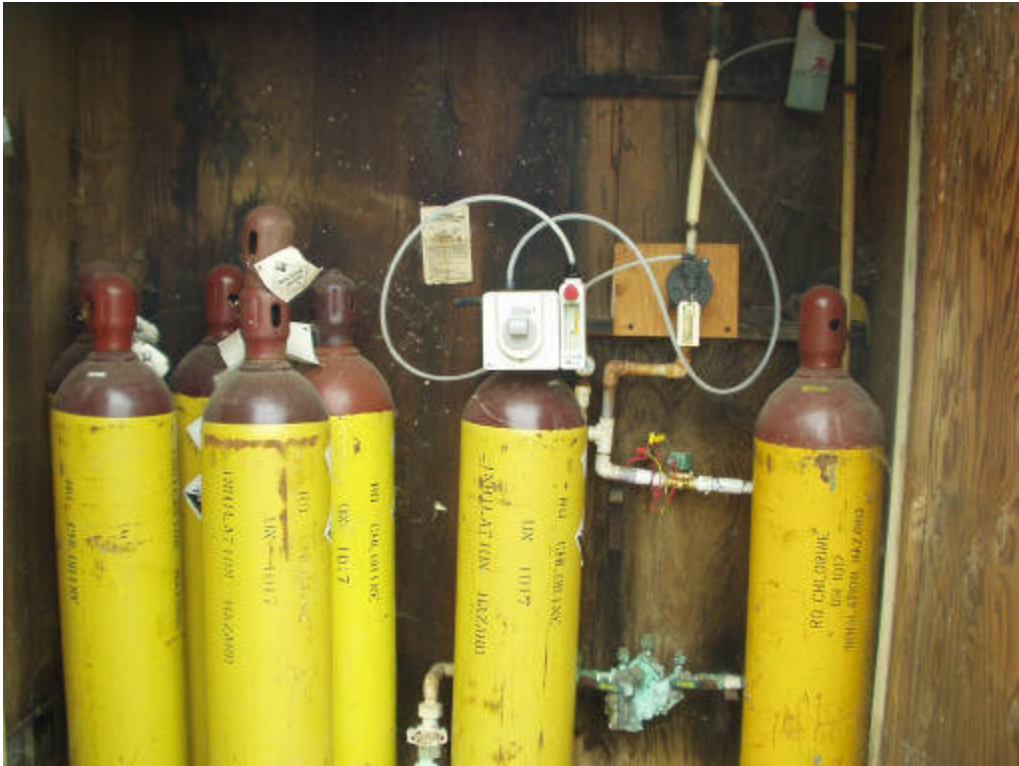
Interior view of the chlorine gas injection system shed.
