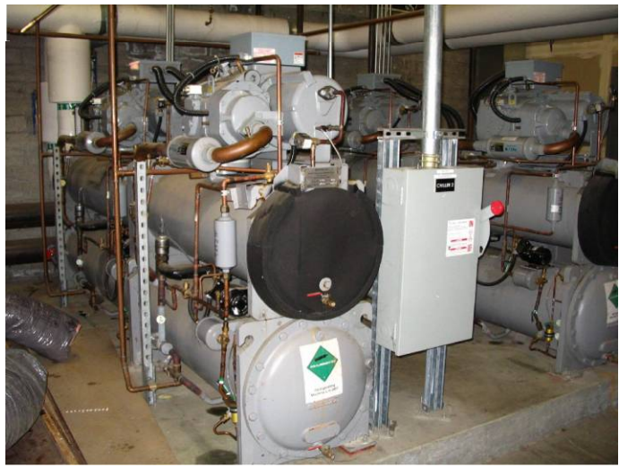
CHILLER ROOM- PHYSICAL PLANT BUILDING
