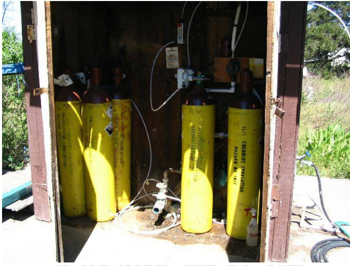
CHLORINE CYLINDERS- WWTP STORAGE SHED
