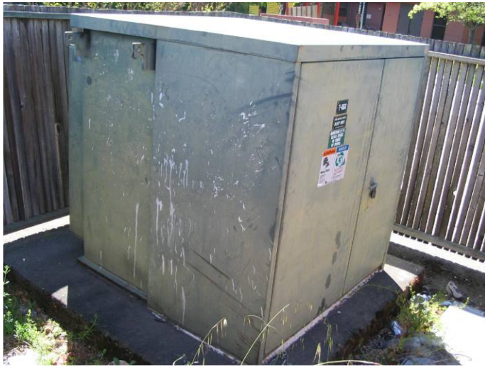
WFC PAD-MOUNTED TRANSFORMER
