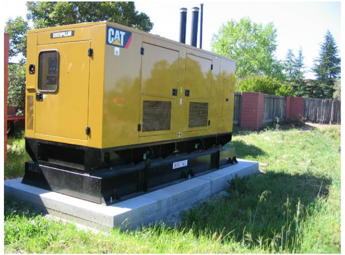
WFC BACKUP GENERATOR WITH BASAL DIESEL TANK
