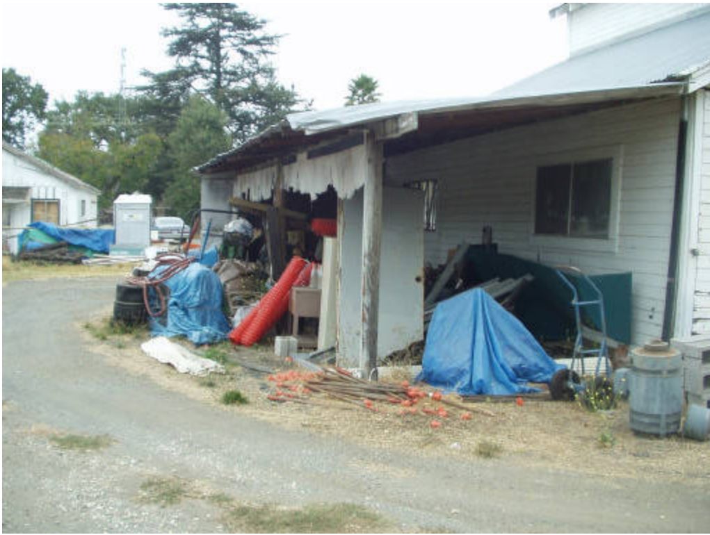
View to the north of storage area on the west side of barn building.
